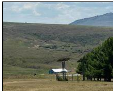
Figure 3-7 Solar panels for pumping water out of the borehole at Ha Nkai
