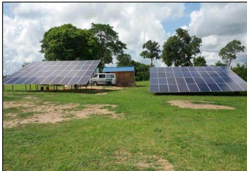
Figure 1-3: Solar PV array 3
