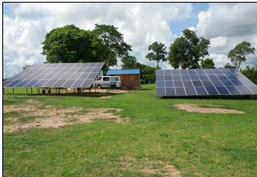
Figure 1- 3: Solar PV array 3
