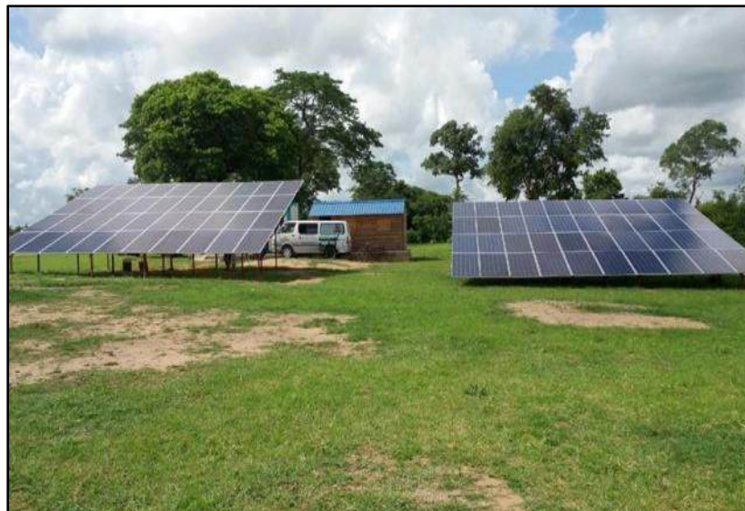
Figure 1- 3; Solar PV array 3
