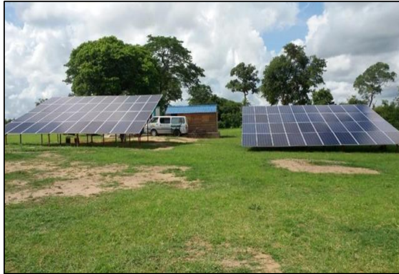
Figure 1-3: Solar PV array 3
