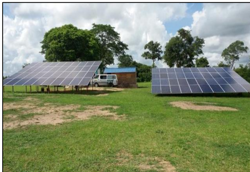
Figure 1-3: Solar PV array 3
