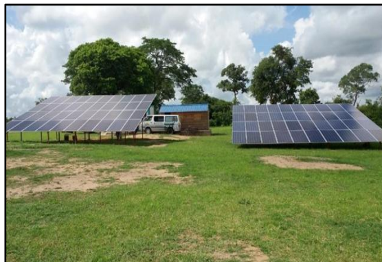
Figure 1- 3: Solar PV array 3
