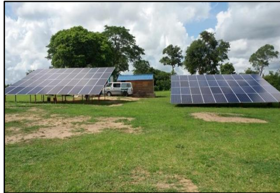
Figure 1- 3: Solar PV array 3
