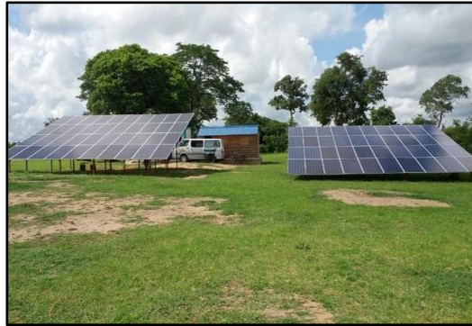
Figure 1- 3: Solar PV array 3
